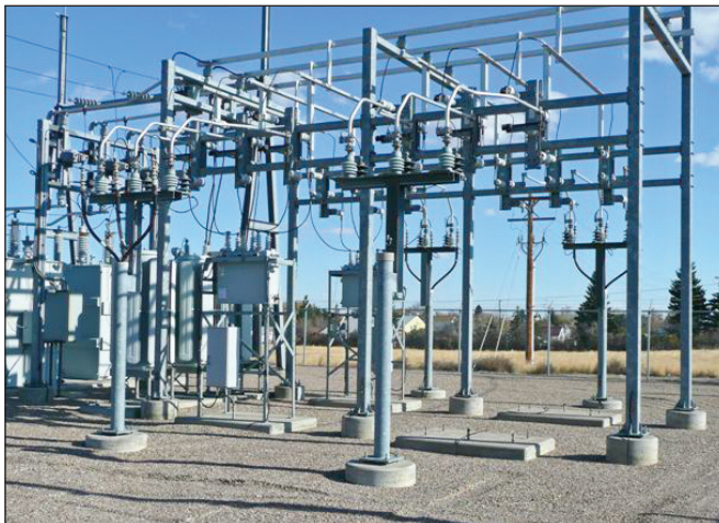
A cooperative substation.
