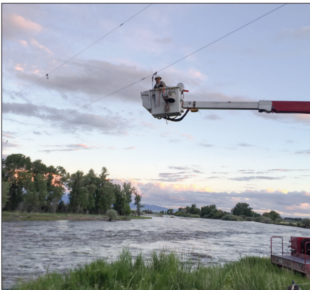
Pictured is Journeyman Lineman Austyn Paulsen. Austyn was part of a crew of linemen who worked to restore power on a section of line crossing the Jefferson River. Due to high river conditions, the bank eroded, taking one of our power poles into the water.
