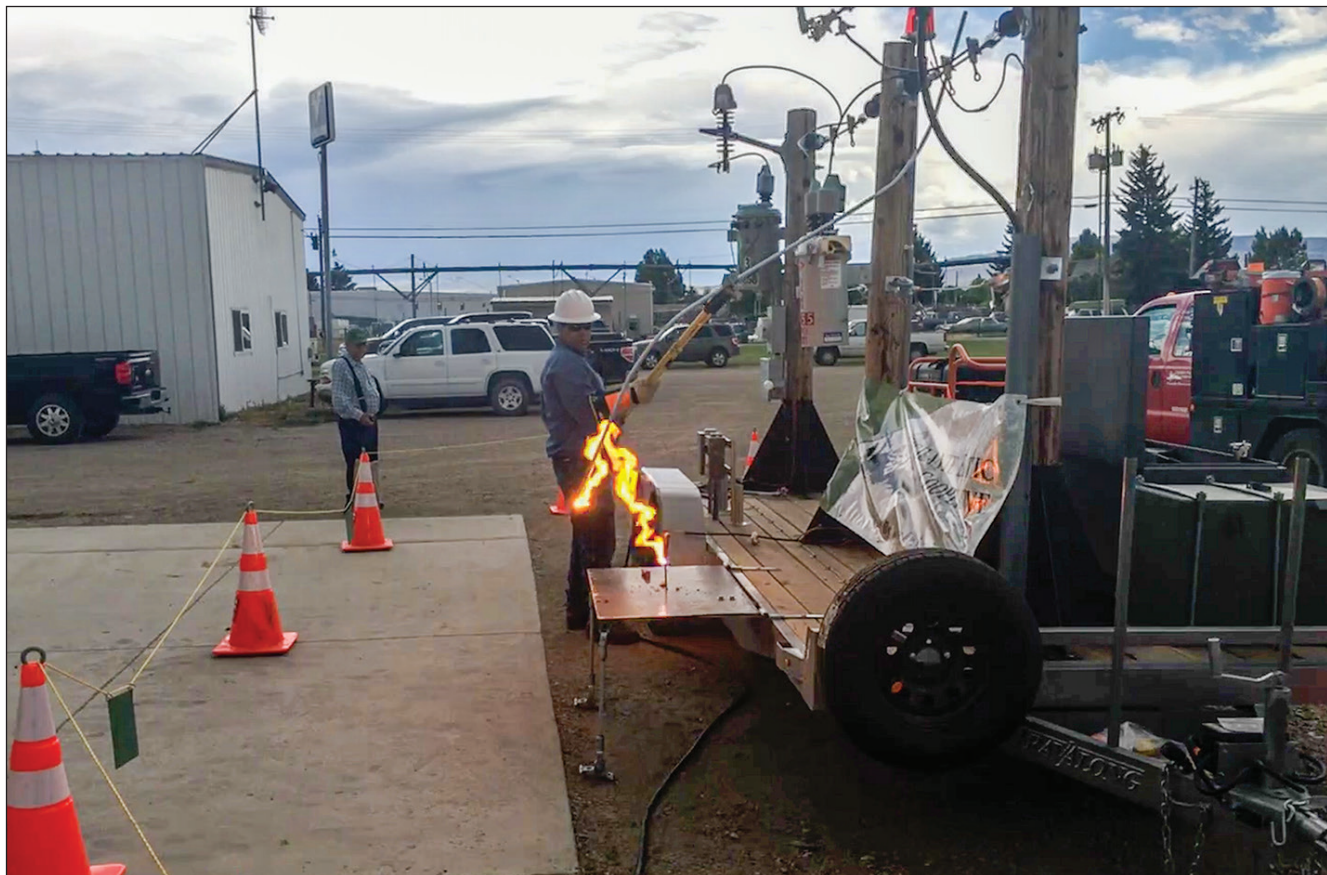
Pictured is Vigilante Electric Cooperative Lineman Cody Tarter handling the hot work for the first safety demonstration done with our new high-voltage trailer.
